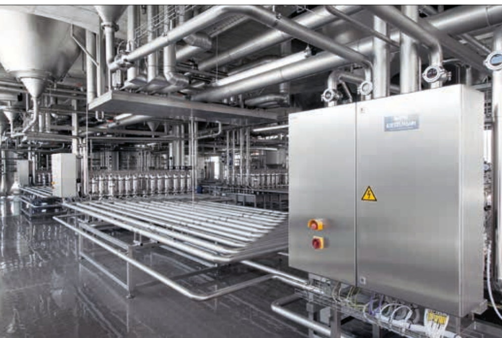
The heart of the matter: the line, three of the eight valve nodes and the ceiling-mounted tanks in the storage cellar
